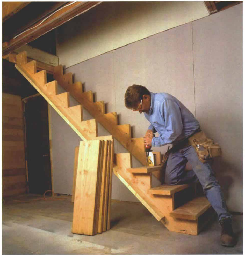
Treads are attached with screws. Screwing the treads to the stringers is the best way to keep the staircase from squeaking. Predrilling the holes prevents the screws from snapping while they're being driven.
