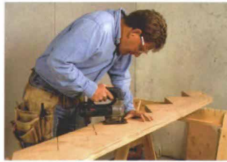
Finishing the cut. A jigsaw is used to complete the cuts in each corner, cutting the wood that the circular saw can't get. A handsaw will also work instead of a jigsaw.
