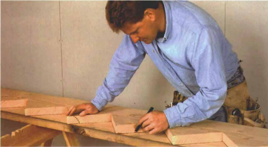
The first stringer becomes a template. Once the first stringer has been cut and tested in place, it can be traced for the layout of the second stringer. The crown of the stringer stock must be facing the same direction as the points on the template.
